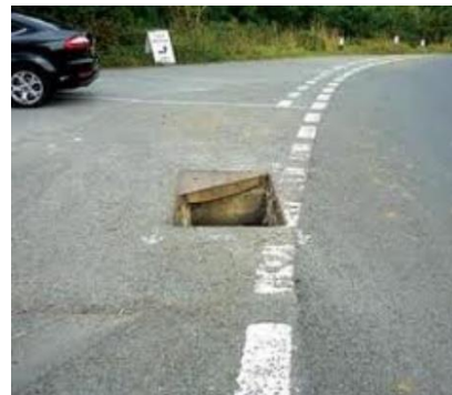
Missing Inspection cover
