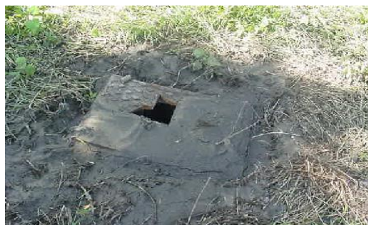
Broken Inspection cover
