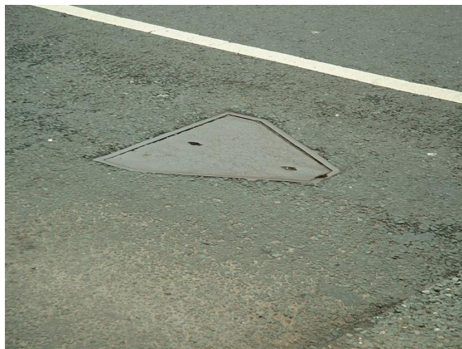
Worn and polished inspection cover
