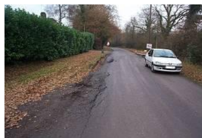
Depression and heave along edge of road
