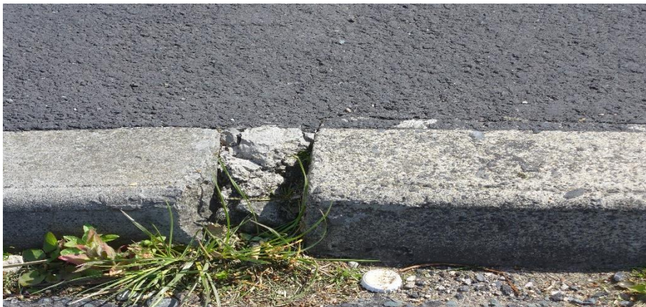
Gap between kerbs
