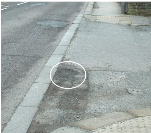
Potholes in pedestrian crossing of side road
