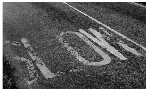
Approx 30% faded markings
