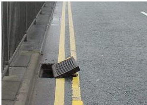
Displaced gully grate
