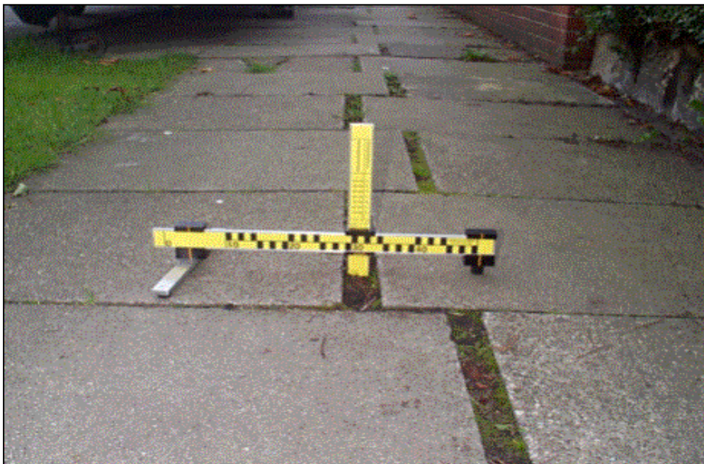
Open joint between paving stones
