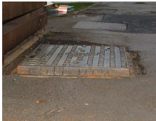
Protruding Inspection cover
