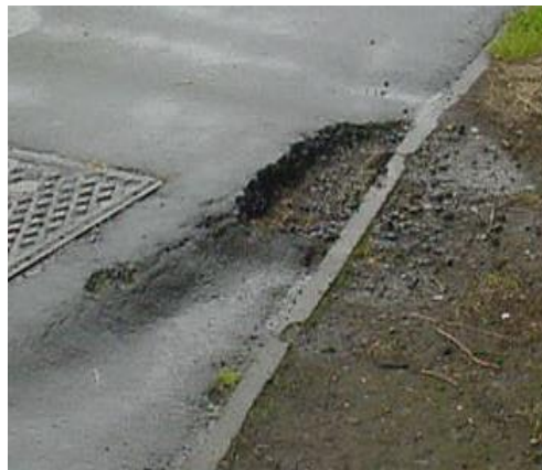
Pothole in footway exposing unbound material
