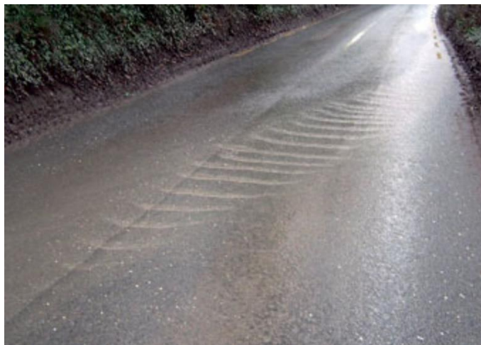
Water flowing across carriageway due to blocked highway drain
