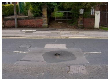
Depression in centre of road
