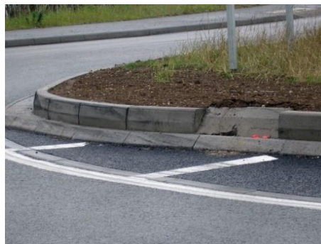
Kerb misaligned horizontally away from carriageway
