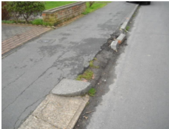
Kerb misaligned horizontally
